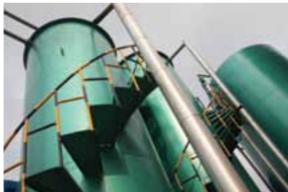
Hi-tech waste-water processing with Biological treatment facility to minimize the environmental impact
